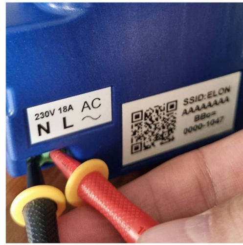
Figure A2 Checking AC voltage
